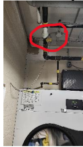
Gas Shut Off picture in laundry
