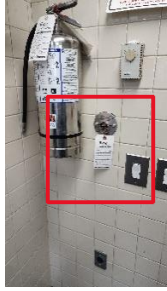
Suppression System picture
